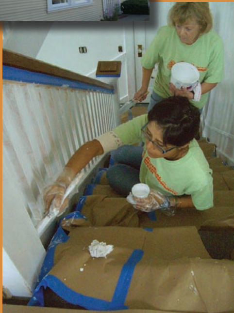
Volunteers painted and revitalized the Tender Life Maternity Home in Ventura as part of NeighborWorks® Week 2008.
